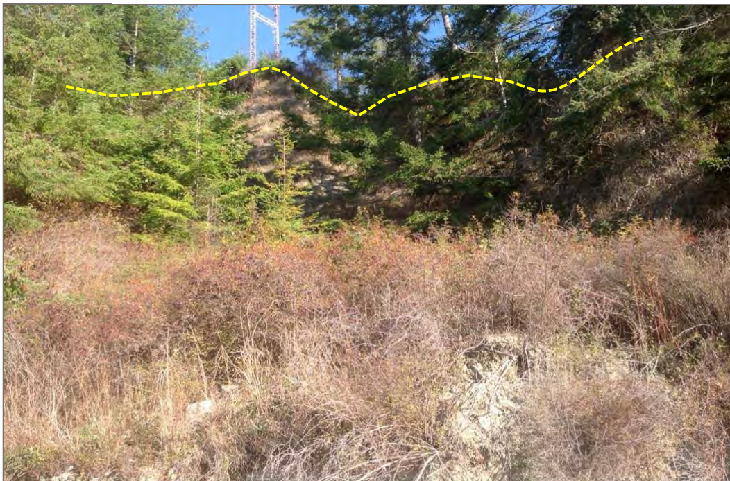
Photo 6: View of coastal escarpment looking up at cable TV tower at the west end of Gillies Bay. Yellow dashed line delineates approximate crest of slope; note v-shaped gully and exposed soil near the crest. (Photo taken October 2016).
