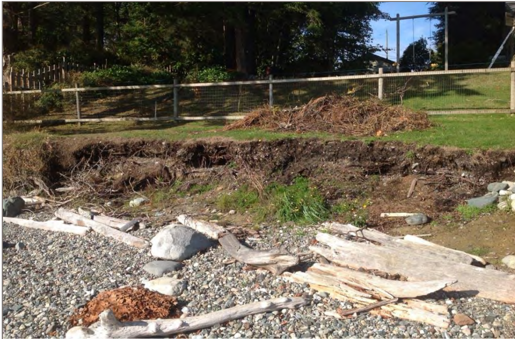
Photo 11: View of coastline erosion along the west side of Gillies Bay. (Photo taken October 2016).
