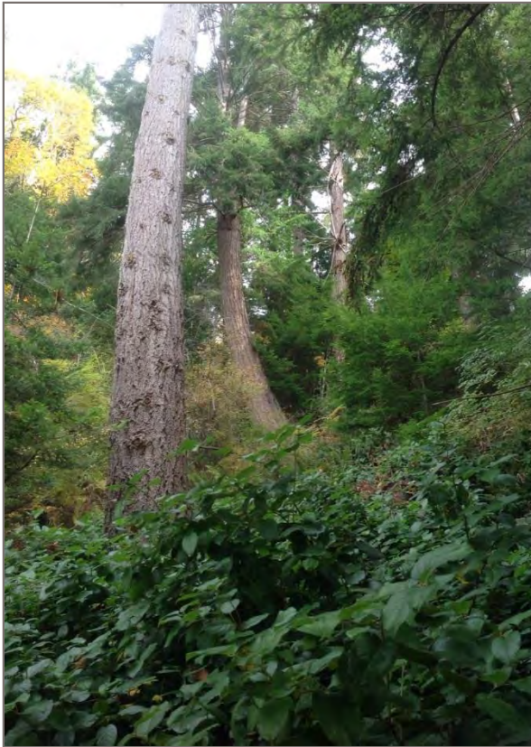
Photo 9: View of coastal escarpment along east side of Gillies Bay. Curved tree trunks indicative of slope creep and potential slope instability. (Photo taken October 2016).
