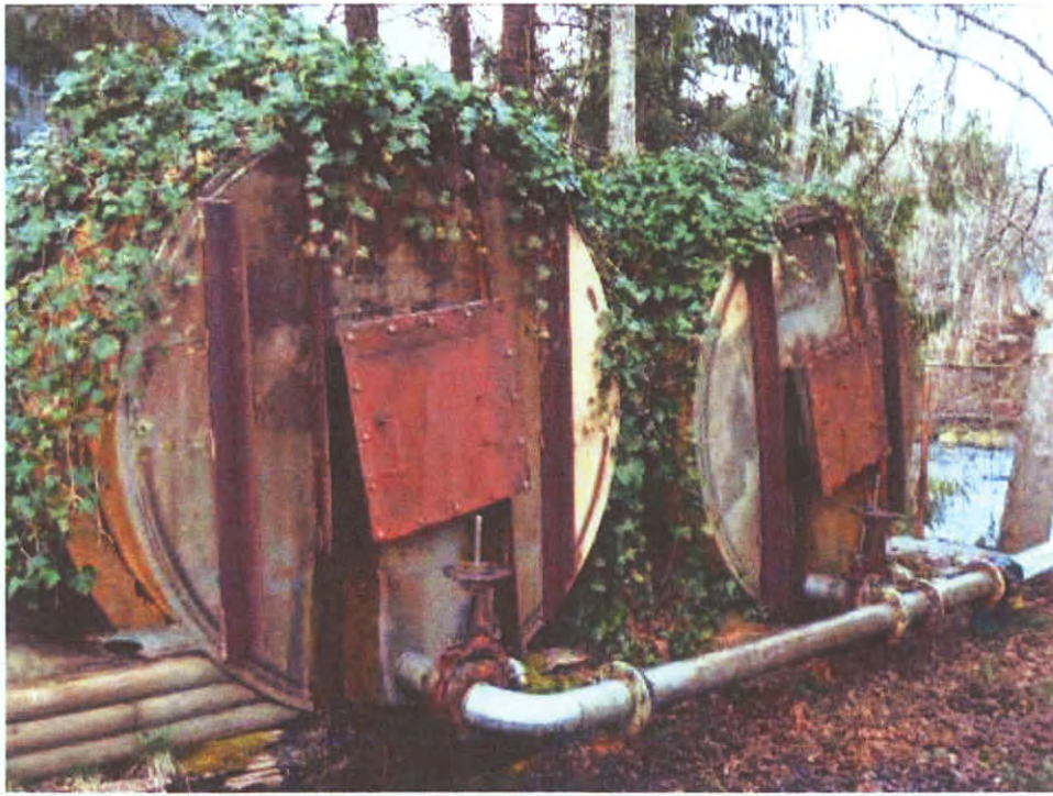
Photo 3: Inlet to Steel Storage Tank
