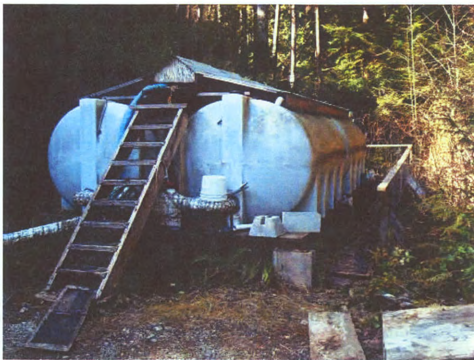
Photo 1: Acrylic Storage Tanks; 4 – 1250 lgal
