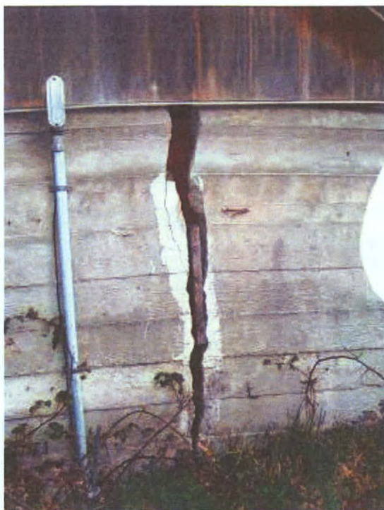
Photo 5: Failed Chlorination Building Foundation
