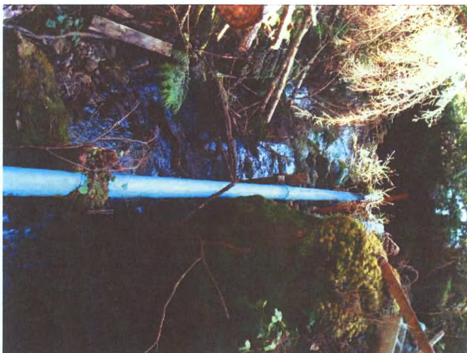
Photo 9: Supply Line from Intake to Storage Tank
