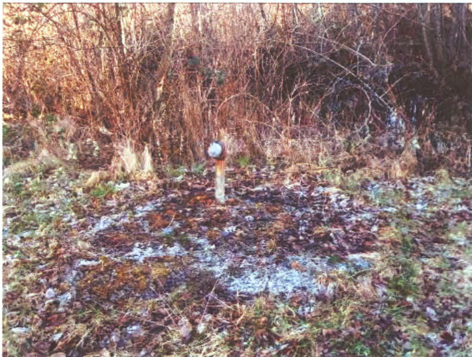
Photo 13: Old Well Pump – now used for Fire Truck Supply
