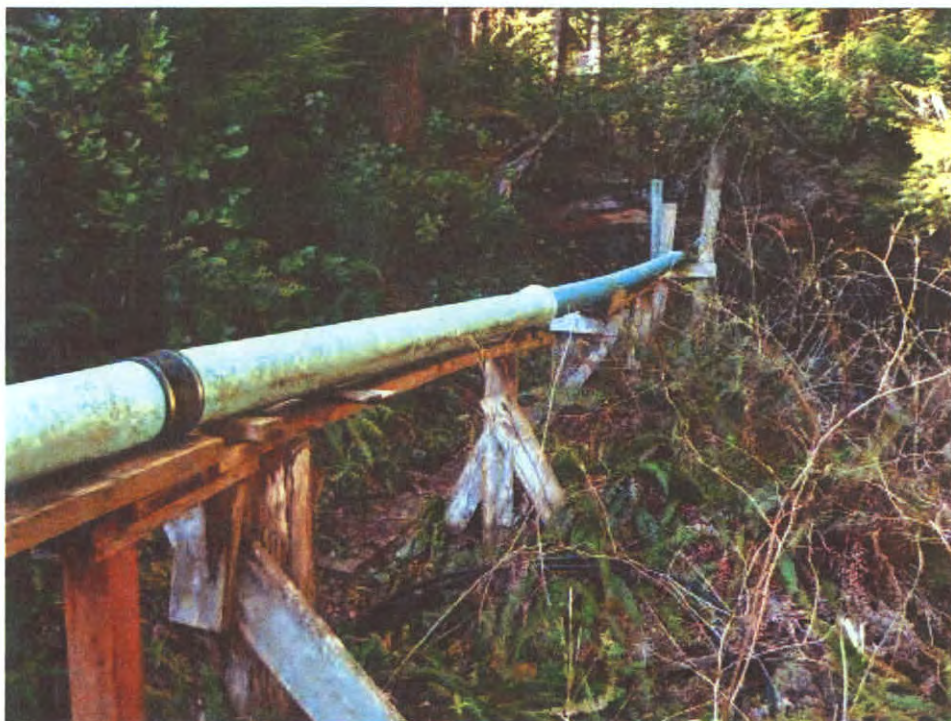
Photo 12: Piping Intake to Storage Tank
