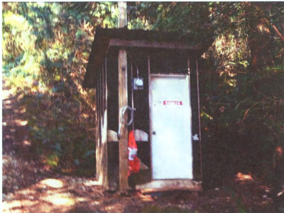
Photo 4: Flow Meter & Chlorination Building
