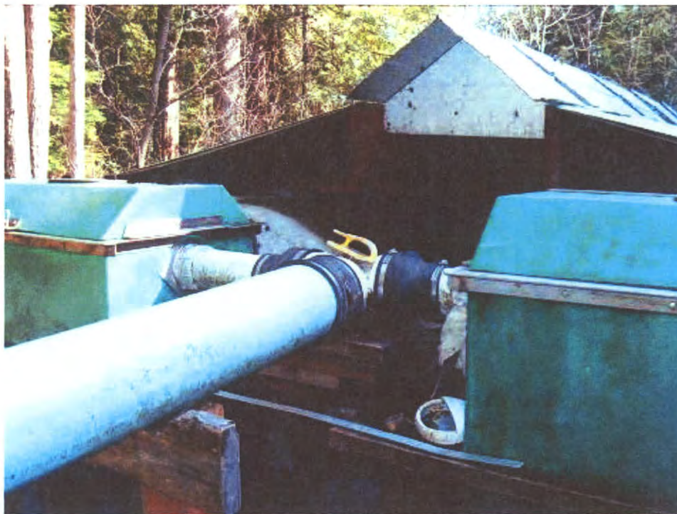
Photo 11: Inlet Header to Storage Tank
