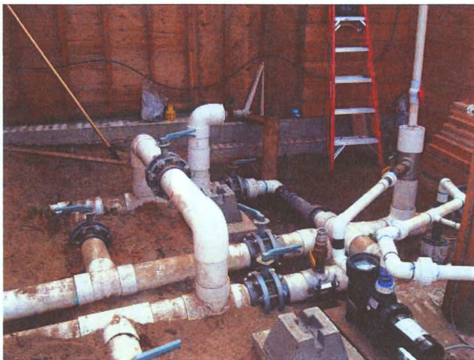
Photo 3: Piping Arrangement – Chlorination Builder
