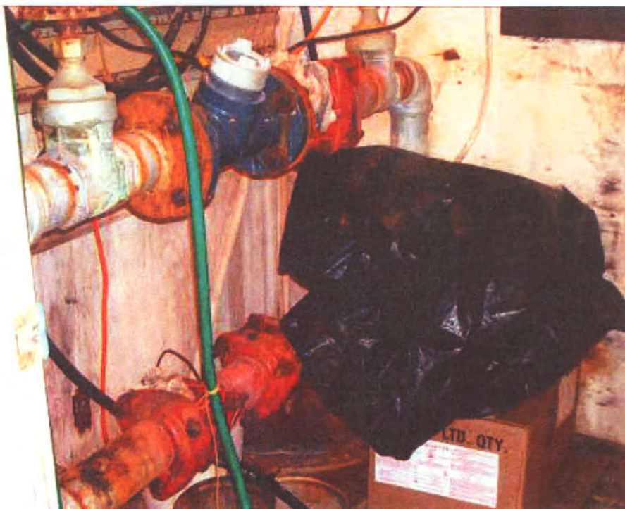
Photo 2: Flowmeter and Chlorination Building
