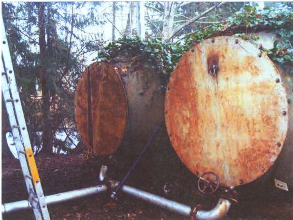
Photo 4: Outlet from Storage Tanks to Pumphouse
