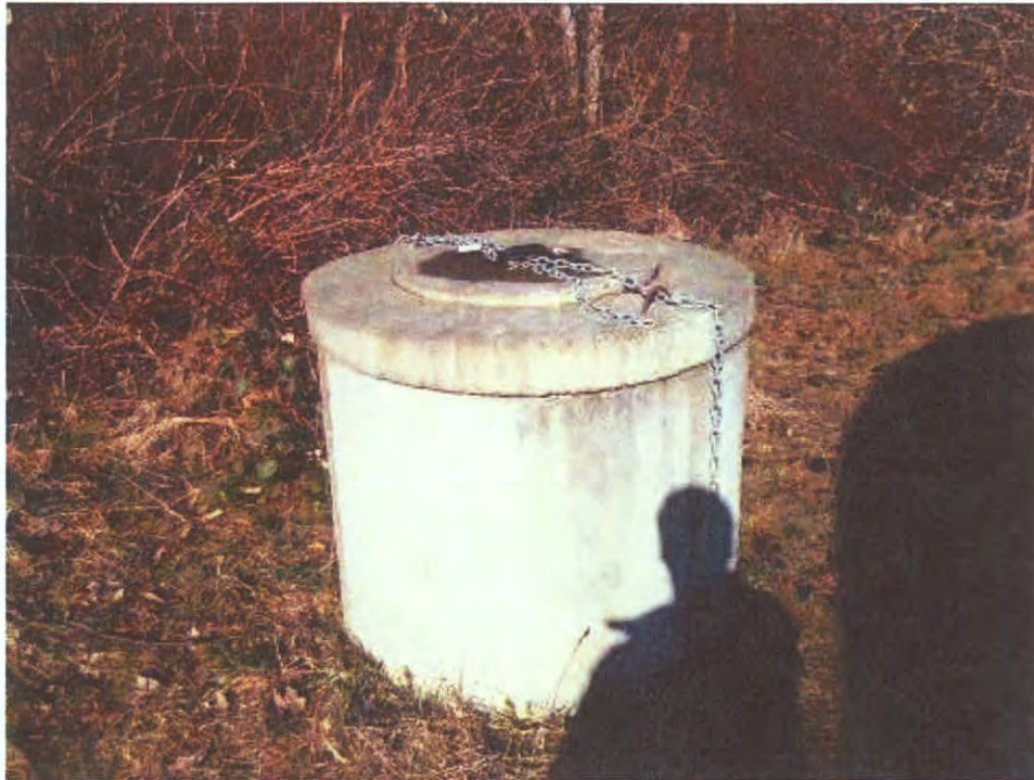
Photo 12: Well Pump Manhole
