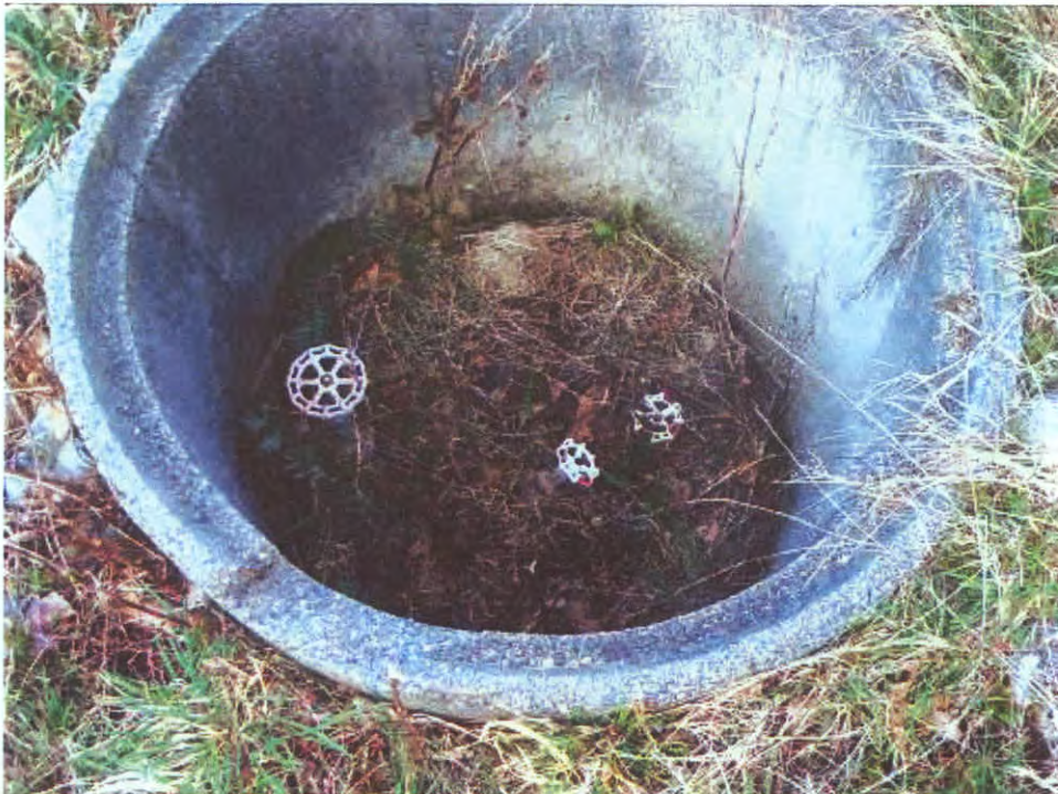
Photo 2: Typical Valves and Manhole for Hydrant Isolation
