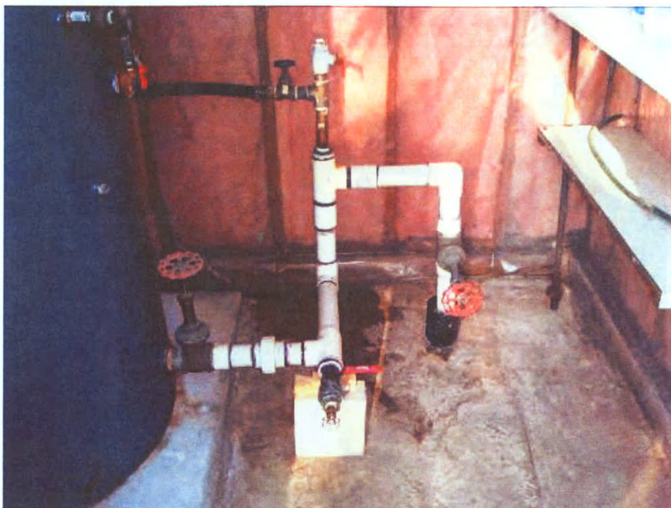
Photo 4: Storage Tank Discharge to 50mm Distribution System
