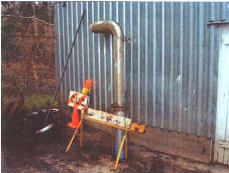
Photo 2: Distribution System Discharge – 60-80psi
