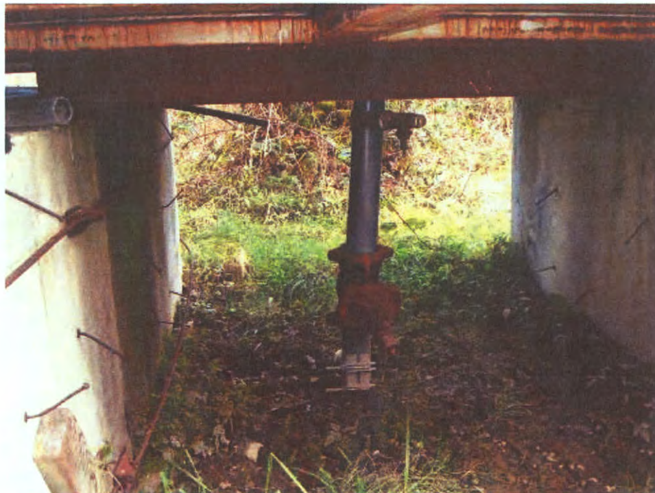
Photo 8: Distribution System Outlet from Storage Tank
