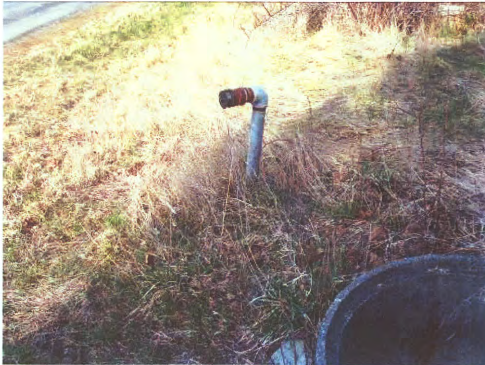
Photo 1: Typical Standpipe Hydrant
