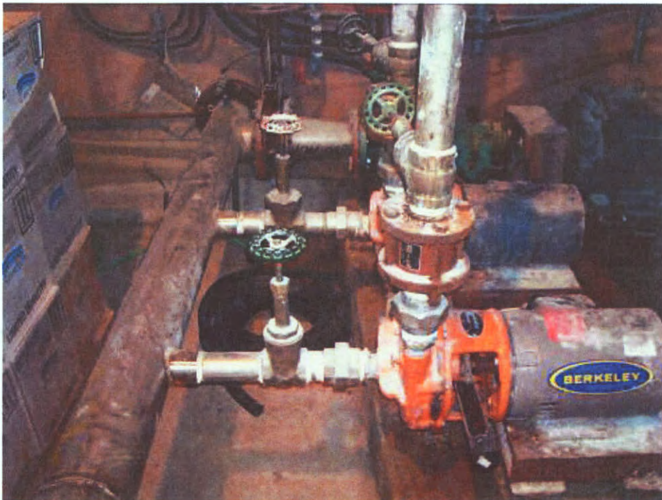
Photo 6: Booster Pumps 2-225 USgpm Berkley and 1-500USgpm Fore
